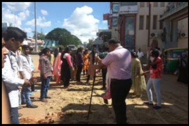
Department of NSS organized Shramadhan on 1 st October 2018, students covered the potholes on the roads with mud
